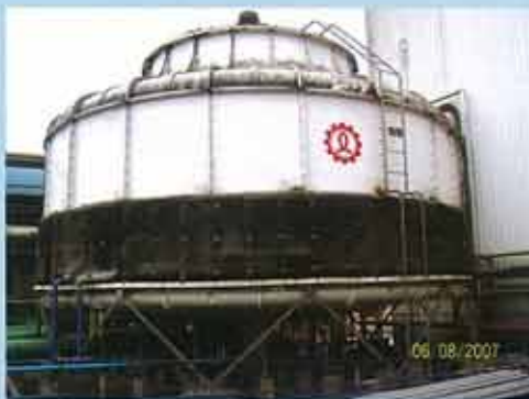
THAILAND THAI POWER SUPPLY LBC-T-1500 X 1 SET
